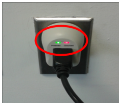
Figure 5 - Picture of Red and Green Lights on the Surge Protector
